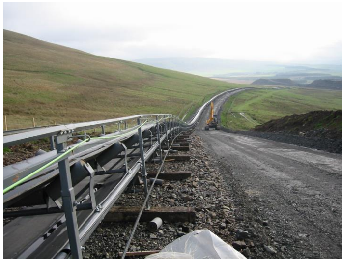
ATH Coal Conveyor which crosses many water courses all of which are monitored by NDSFB.
